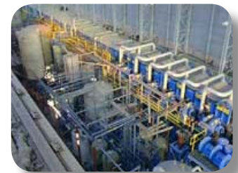
Ideal for Steel Pickling operations and much more...
